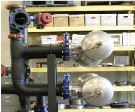
Figure 1: Inlet/outlet piping support
