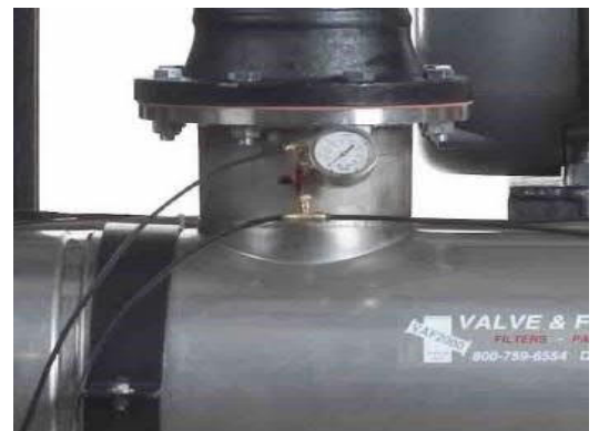
Figure 6: 3-Position manual valve and pressure gauge
