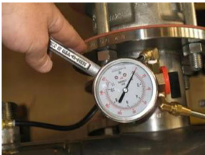
Figure 31: Removal of pressure gauge
