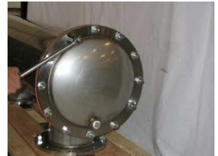
Figure 10: Removal of lid
