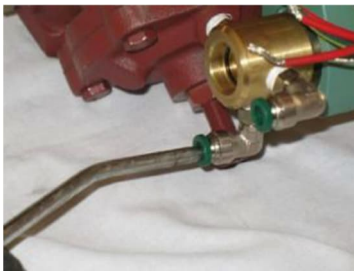
Figure 46: Blowing out the solenoid supply lines.
