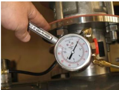
Figure 39: Removal of pressure gauge
