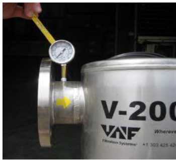
Figure 19: Removal of pressure gauge
