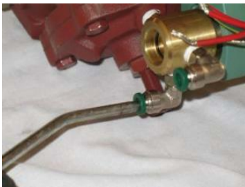
Figure 38: Blowing out the solenoid supply lines
