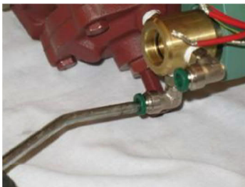
Figure 25: Blowing out the solenoid supply lines
